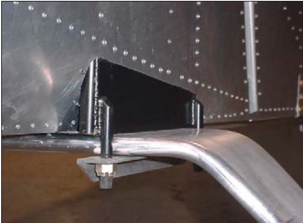
Cutout in the side skin is below the diagonal rivet line.
