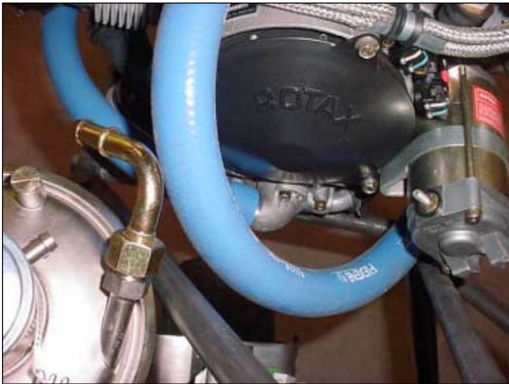
90 degree elbow on the water pump at the back of the engine (at center of photo).
