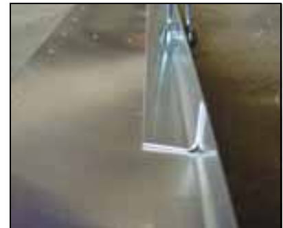
6T1-6HD clamped to the top flange.
