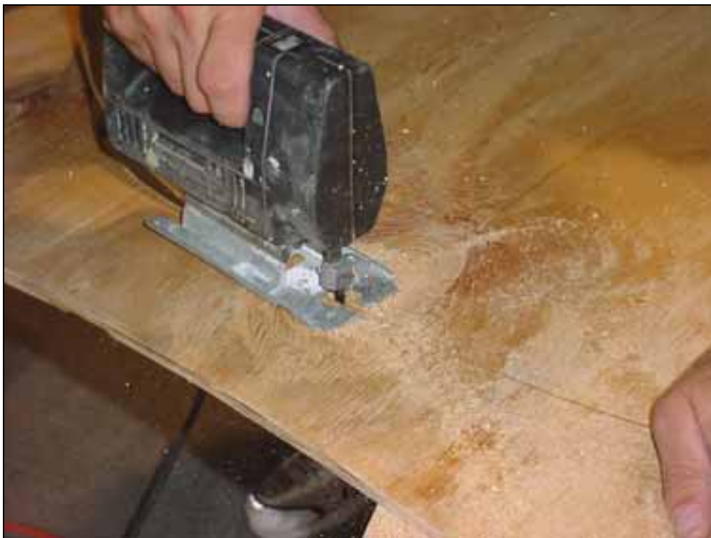
Use a jig saw to cut on the line. The critical part is the outside blank, if you have too cut small on the inside of the line, then go back and cut on the line.
