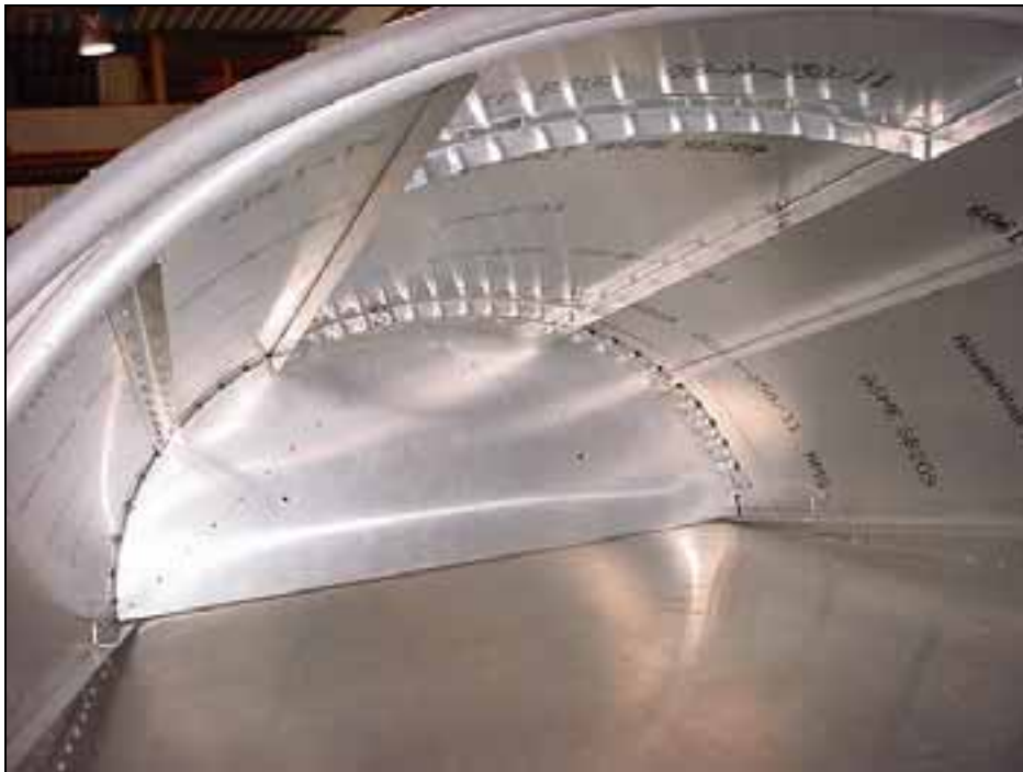
Crimped L angles between the two middle L angles for antenna reinforcement
