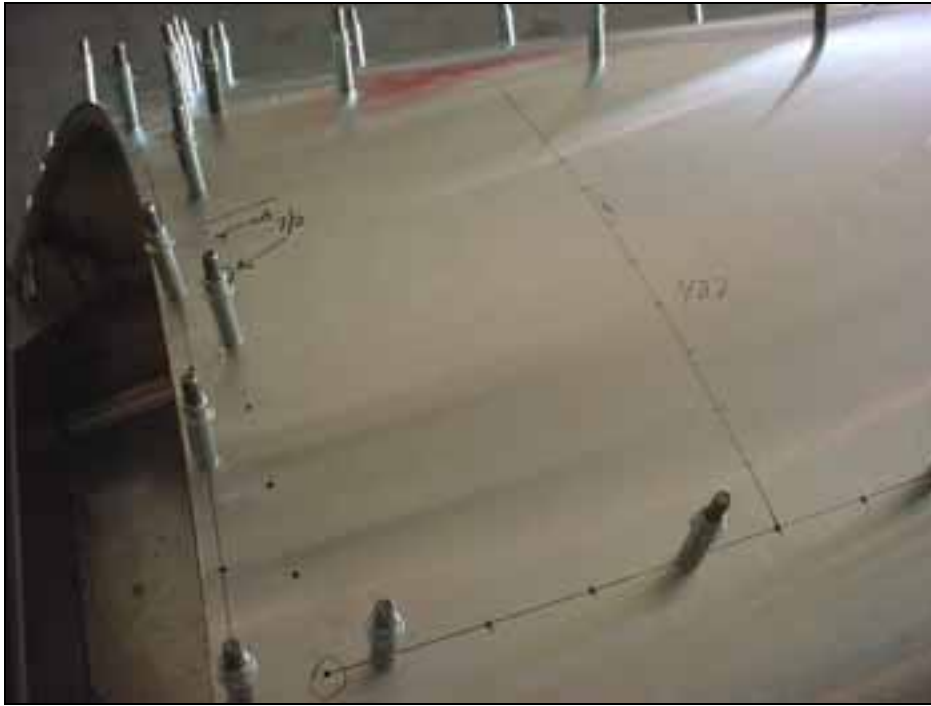
Location of crimped L angle for antenna support.
