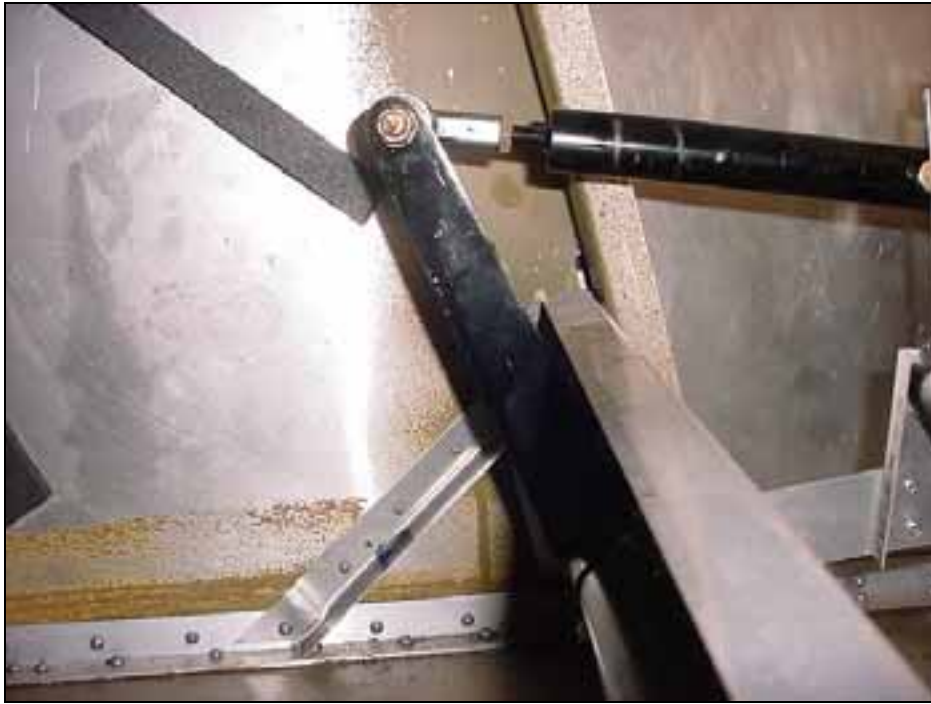
Detail of the flap control arm 6B19-3 in the flap up position. CHECK: There is some clearance between the front of the arm and the aft edge of the rear frame channel 6B5-2
