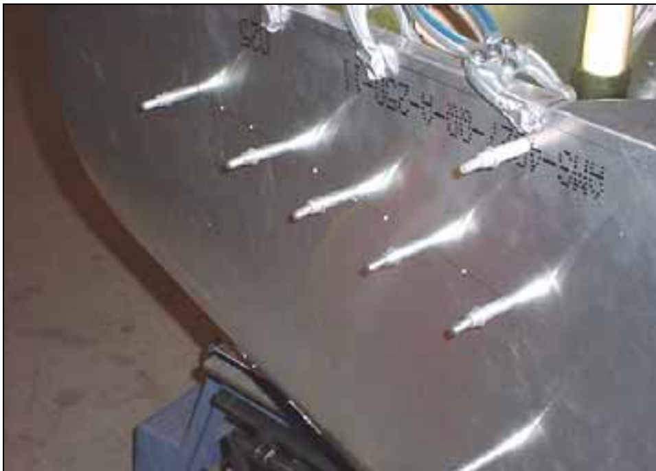
Lay out the rivet across end holes. Layout the rivet pitch. Drill an end hole in L angle, cleco in place and back drill end hole through firewall flange.
