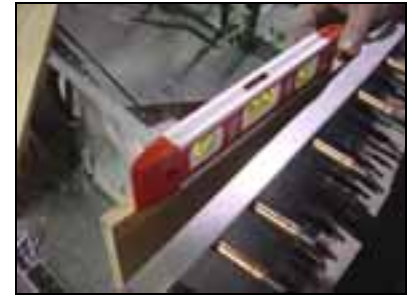
The Plywood spar template is square to the gear channel; it is not in line with the fuselage sides.
